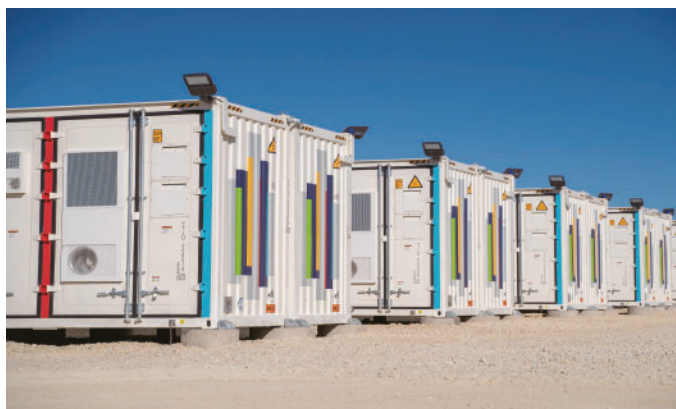
Texas, USA – regulace frekvence, 226 MWh
